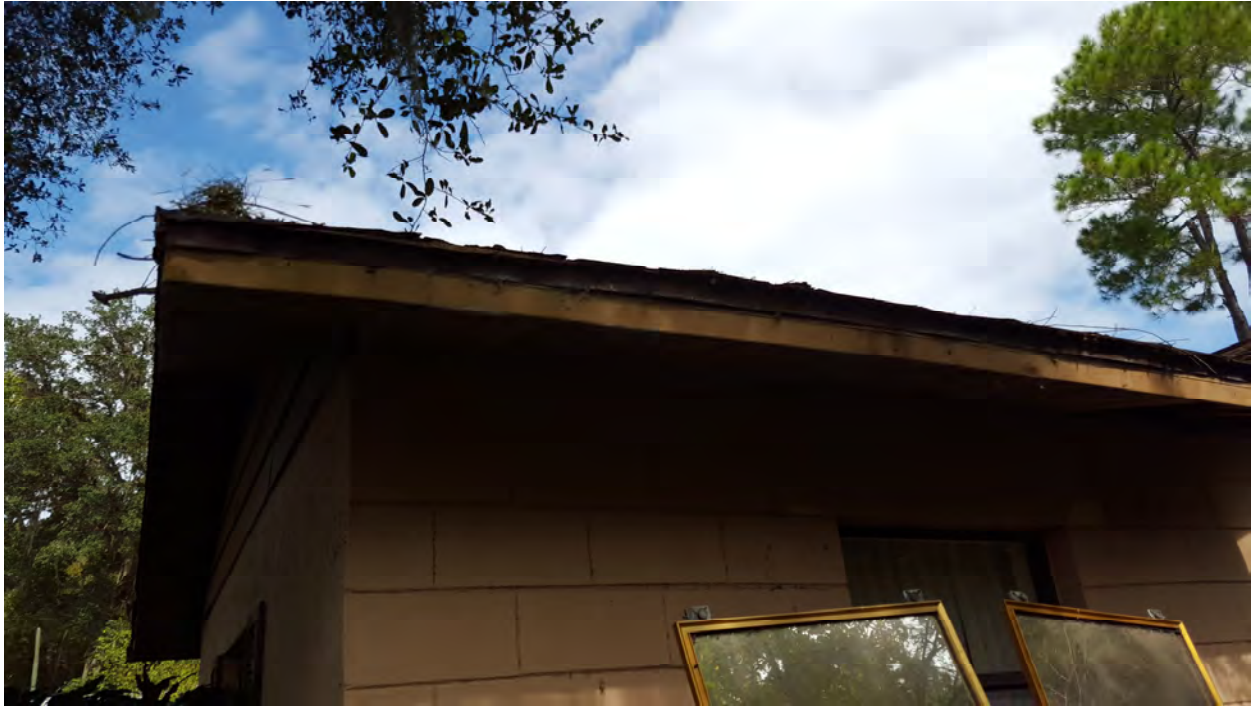
Figure 3 : Subject residential property showing storm damage resulting from falling limb.
